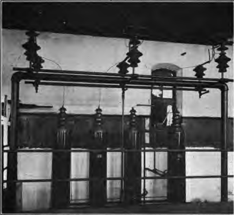
GENERAL ELECTRIC LIGHTNING ARRESTER MOUNTED IN SUB-STATION AT ISHPEMING
